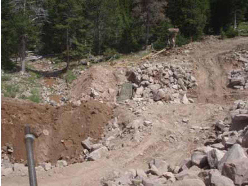
Figure 10: UCC crew assisted in placing the fourth gabion cut-off wall. The third gabion cut-off wall was not installed due to hitting bedrock at its location.
