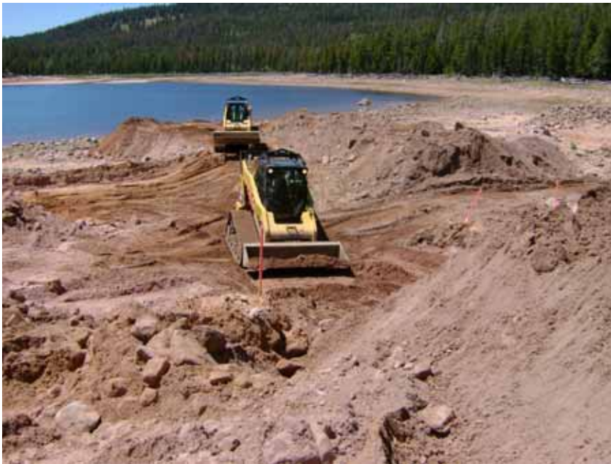
Figure 5: Reclamation crew using skid steer to begin cutting breach through the dam.
