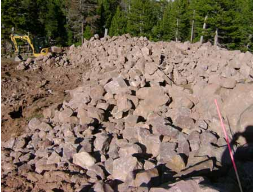
Figure 6: Reclamation crew continued cutting through dam using two mini-excavators and one skid steer.
