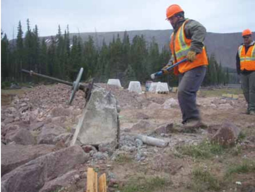
Figure 12: UCC crew using sledge hammer to break up concrete and remove the wheel works and vent pipes.
