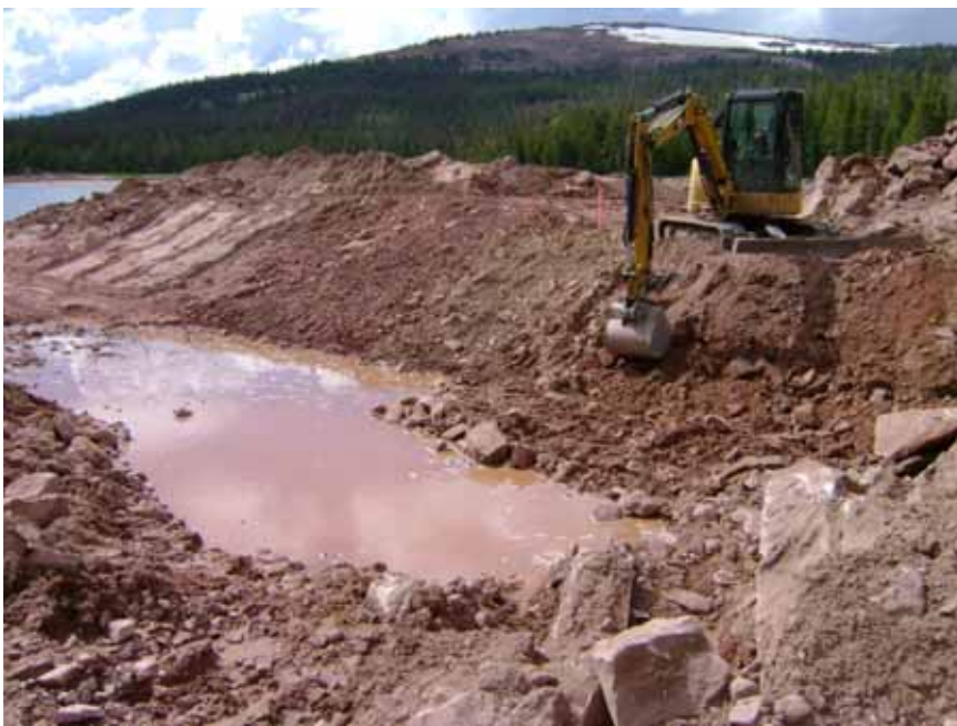
Figure 7: View of breach prior to placing cut-off walls and riprap.
