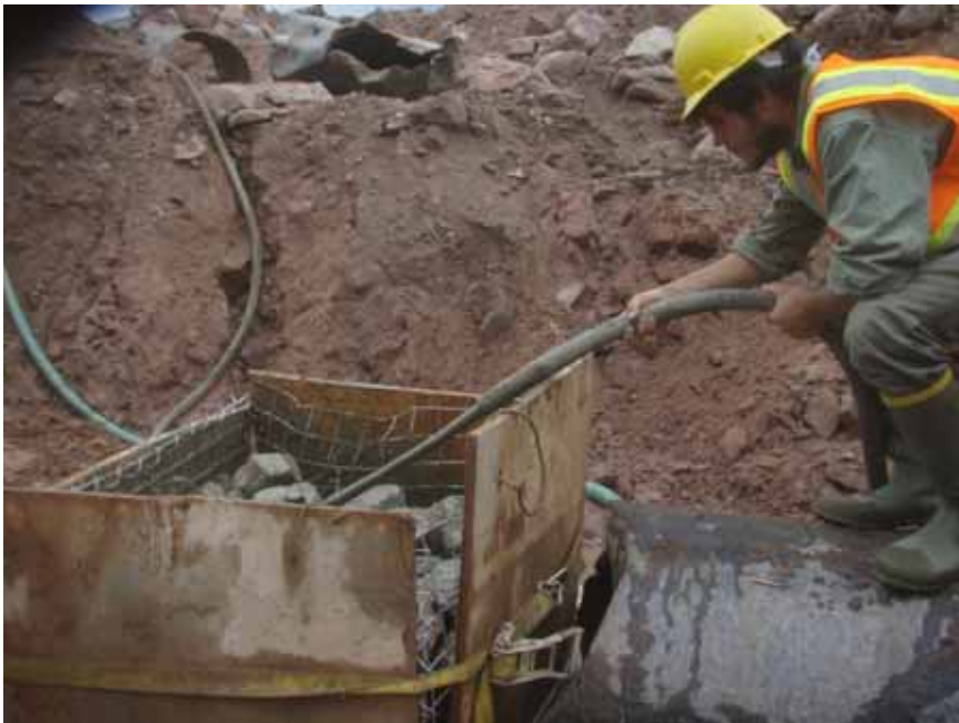
Figure 14: Gabion basket installed at each end of outlet pipe and filled with grout.
