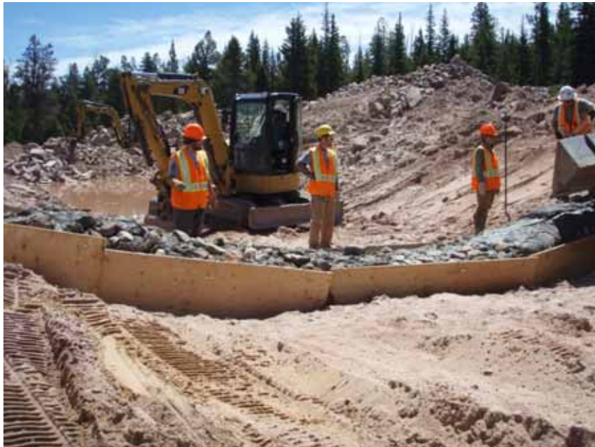
Figure 8: UCC crew helping with installation of gabion baskets at upstream cut-off wall.
